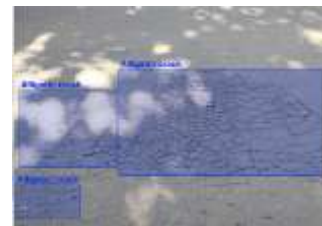
c. Alligator crack
